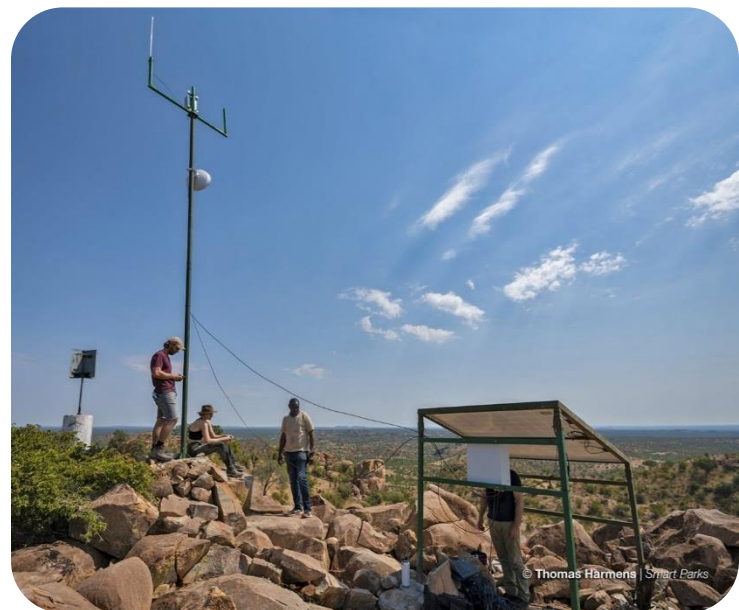
A LoRaWAN tower being erected in the Central Tuli Block, a conservation area in southern Botswana. © Smart Parks
